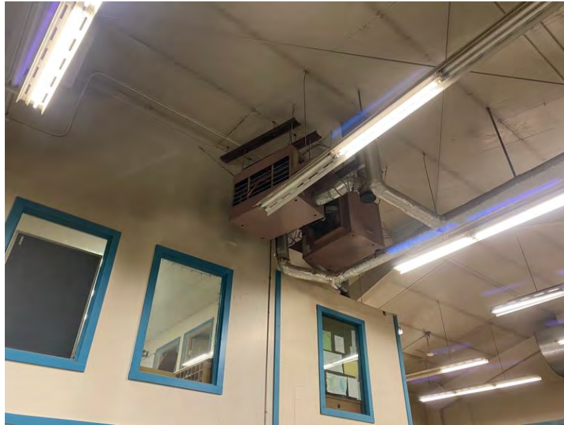
Figure : The unit heaters that heat the vehicle bay are located at roof level and thus much of the heat that they produce is lost to the roof without reaching the floor level where the heat is required.
