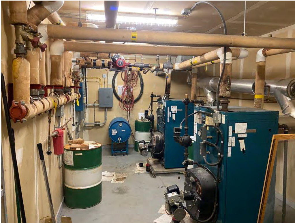
Figure 1: Two large 141.55kW oil boilers heat the Administration Building. The controls cabinet for the building is in the blue cabinet on the left side of the image.
