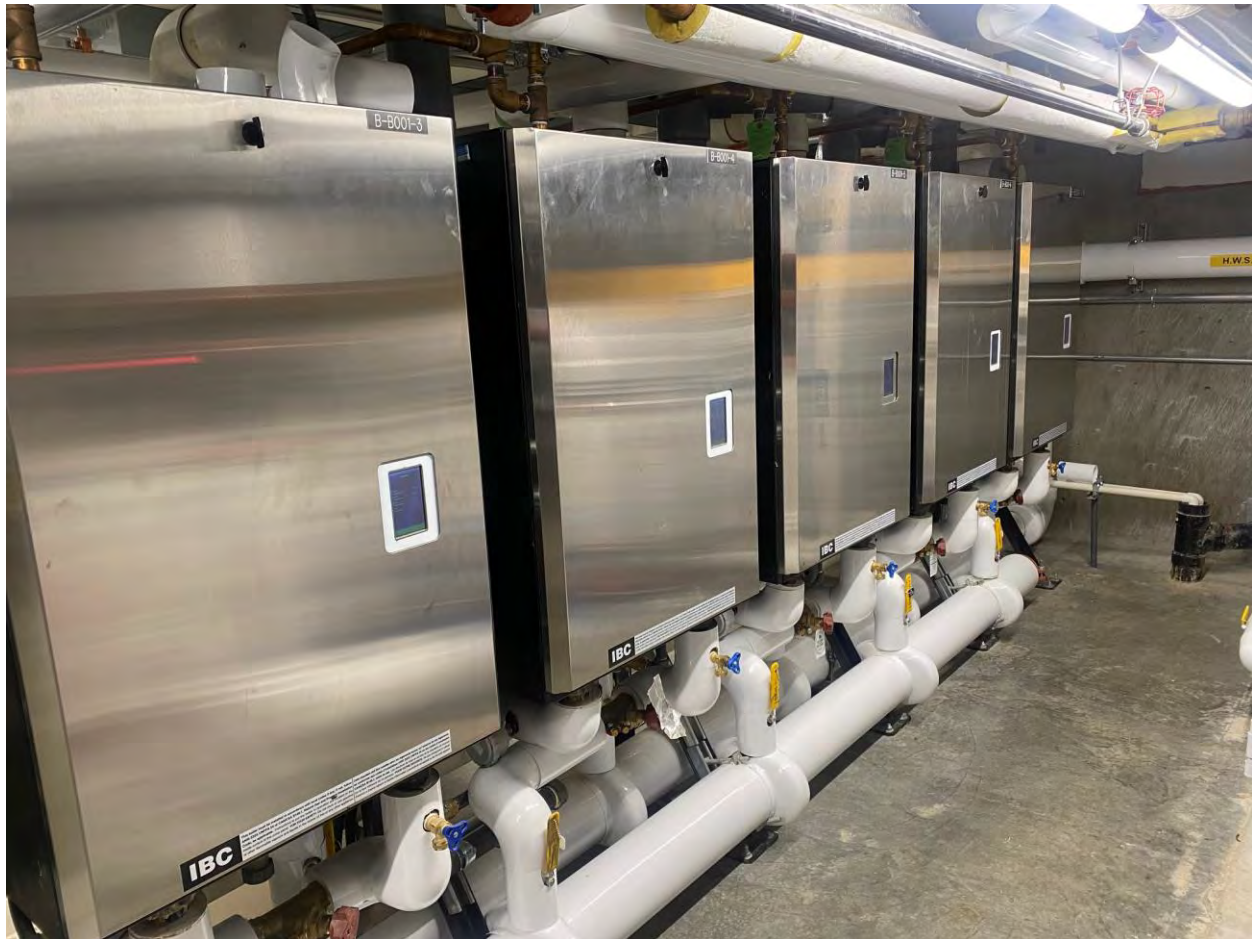
Figure 8: High efficiency propane boilers (IBC SL 80-399 TI Condensing Boilers) used in the Carcross Learning Centre are 95.7% efficient and have a CSA rated output of 22.6kW – 112kW (77 – 382 MBH) per boiler. Based on the current boilers at the Administration Building, it is assumed that 3 of these propane boilers would work well with a biomass system or as stand alone. Since these boilers can be modulated significantly, their implementation would reduce the usability of a heat pump in replacement of the existing air conditioning equipment. They would also work much better than oil boilers for supplementing the performance of a biomass system.
