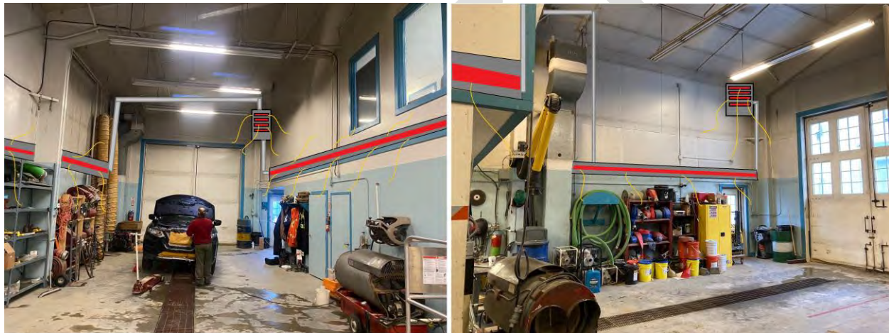
Figure : Radiant wall heating from the biomass system could be run extensively within the public works building in combination with unit heaters that utilize the hot water loop. The unit heaters would ideally be controlled via a secondary thermostat that allows them to boost heat within the space as required when the radiant lines cannot keep up. Insulated hot water lines are shown in grey. Note that the hot water lines from this system could be tied into to provide heat to the second floor via radiant ceiling panels for option 2.1.3.
