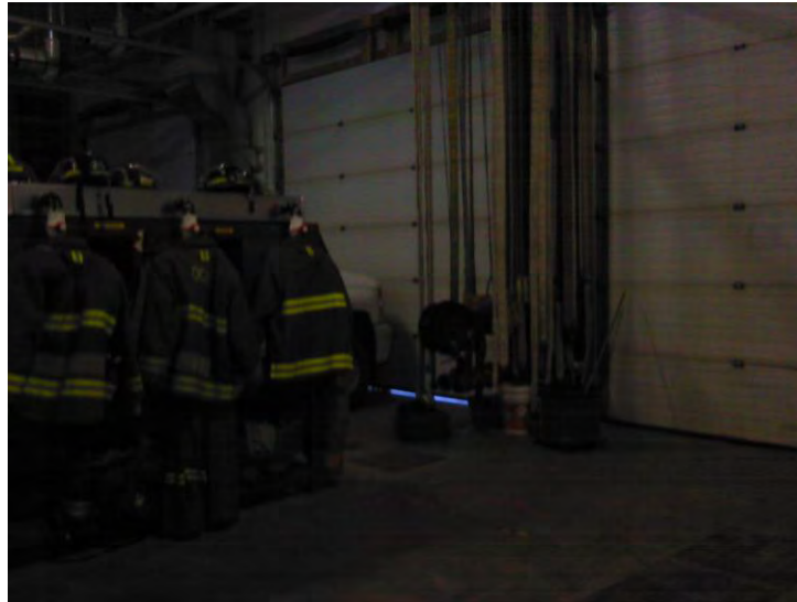
Figure 6: The middle rear bay door appears to have light shining through it at the bottom. The thermal image on both the interior and exterior indicate that a significant amount of heat is escaping through this door.
