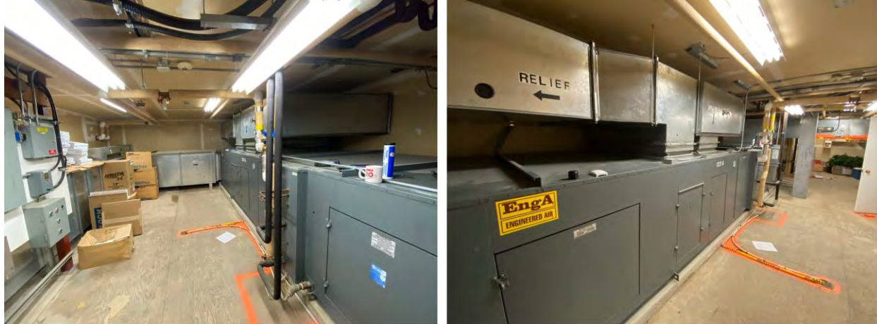
Figure 2: View of the AHU from both sides. Note the marked drain line on the floor for reference.
