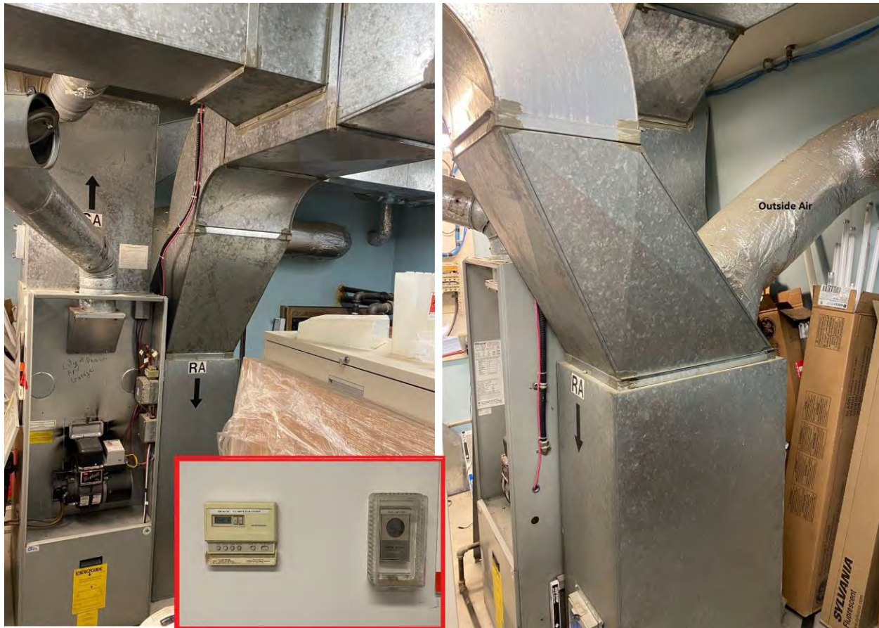
Figure : A compilation of images of the furnace. Left Image: Front view showing the motor and controls. Right Image: Side view of the furnace showing return air ducting with outside air ducting connected. Inset: Thermostats that control the furnace located in the superintendent office.
