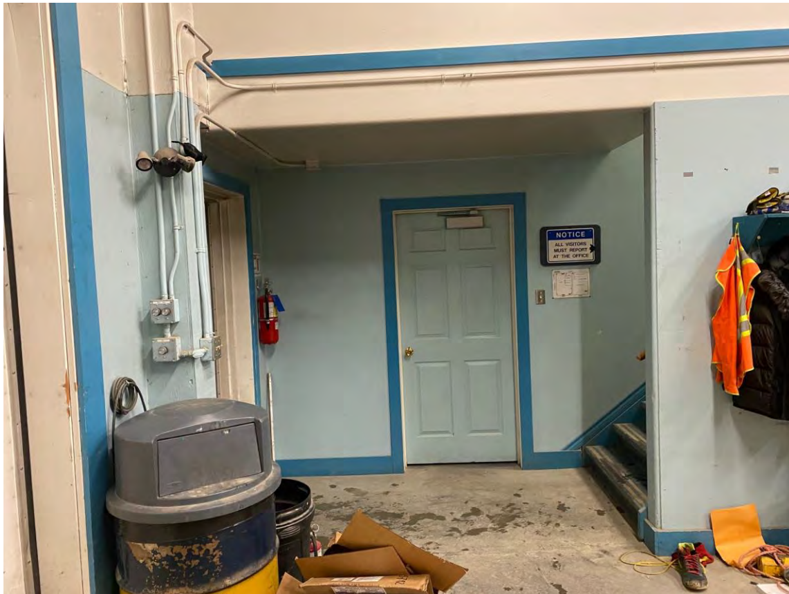
Figure : The open corridor to the upstairs that connects to the vehicle bay can be framed with a door installed to prevent cold air and fumes from migrating upstairs.
