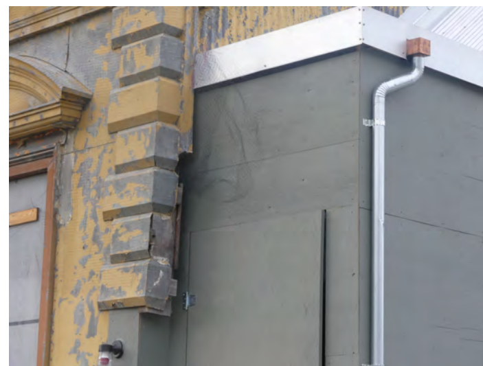
4. north east corner at new stair. The quoins on the north wall are a consistent length of 7" (178mm), with an existing metal filler between the metalwork and the stair structure.
