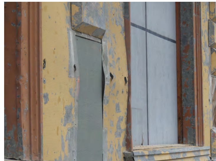
20. area adjacent to entry door, damaged metal molding for door frame, holes in metal siding, damaged sill. This also shows the metal filler strip between each quoin
