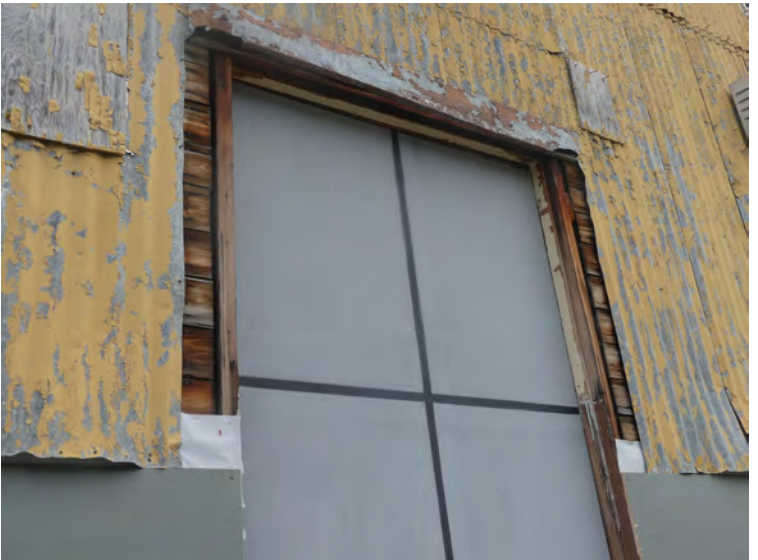
42. lower floor, sill and metal frames to be replaced
