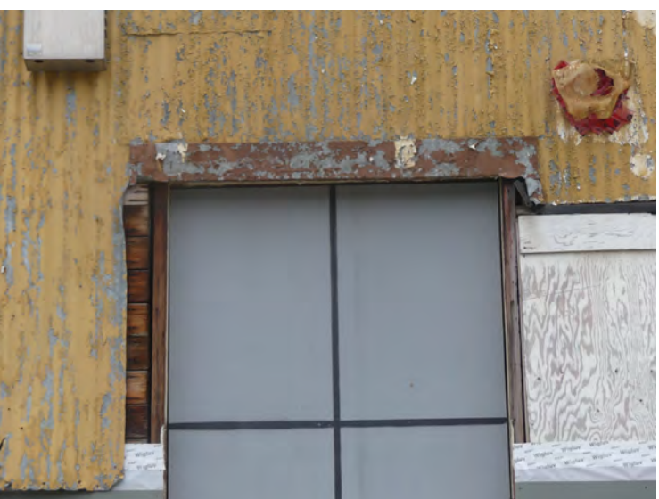
43. window frame, main floor, repair would be straightforward, the chimney thimble would remain
