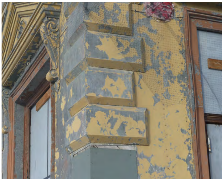
2. south east corner, quoins removed below this level. The taped opening for the chimney thimble (top center) could be retained, with a correct metal closure in place
