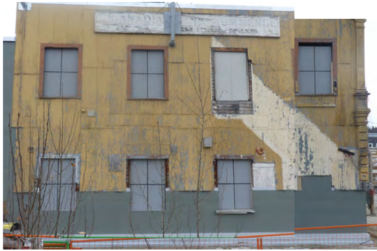
34. west elevation, note changes to framing and the outline of the added stair. The patch below the upper windows indicates the original balcony location and size.
