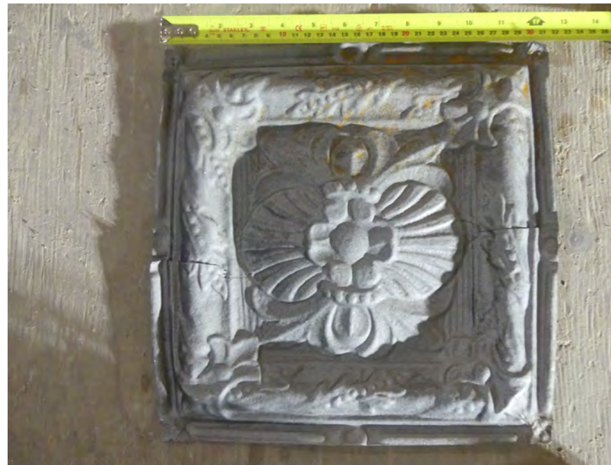
D. intersecting beam panel: 11 1/2 x 11 1/2 net size, 12 1/2 x 12 1/2 overall size total number of panels required: panels available in usable condition: replacement panels required
