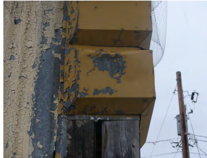
13. south west corner, some of the metalwork is damaged, repair would be feasible as this piece will be removed as a sample
