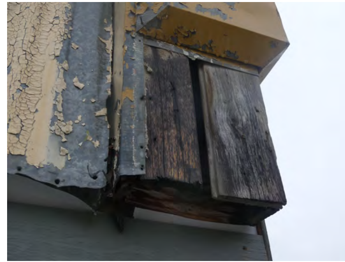
12. west wall, these quoins are all the same length, 12" (305mm) on this face. A typical piece should be removed as a template. This shows the transition to the corrugated metal wall finish, and the wood substrate. Any new backing would be constructed from PT material
