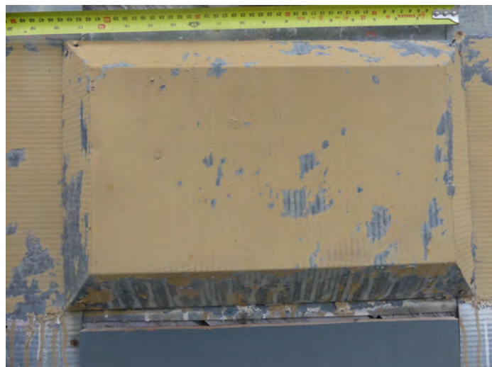
11. the quoin below has been removed, the horizontal transition strips and the condition of typical siding show clearly. Renailing and filling of mail holes and other penetrations will be required
