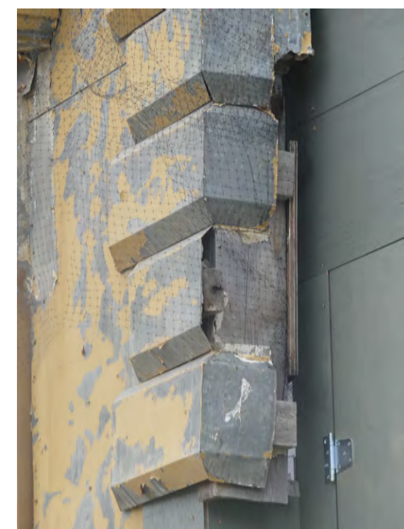
7. detail of damaged metalwork and wood substrate. The new wall will be clad with corrugated metal
