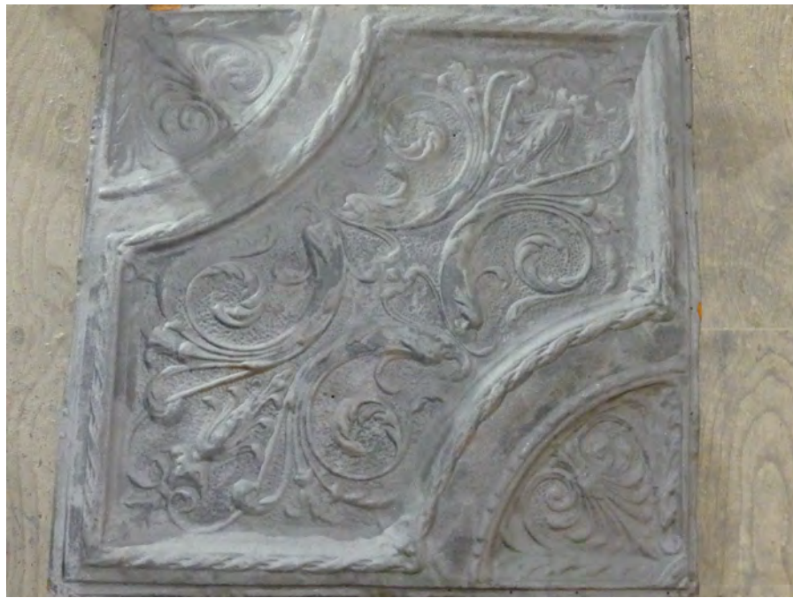
A. typical ceiling panel, 23 1/2 x 23 1/2 net size, 24 1/2x24 1/2 overall size total number of panels required: 9x16: 144 panels available in usable condition: 78 replacement panels required: 66
