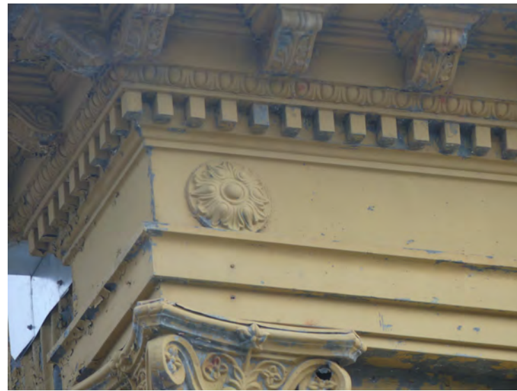
24. detail of remaining medallion, north west corner. This should be removed and replicated for other locations where missing
