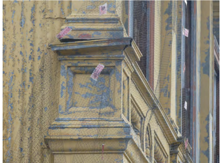
38. metal capital, joints have failed, a decision would need to be made whether to remove to repair, or leave in place
