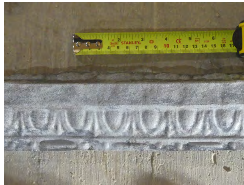
J. egg and dart molding, approx width 3" total lineal footage required: all pieces to be replaced
