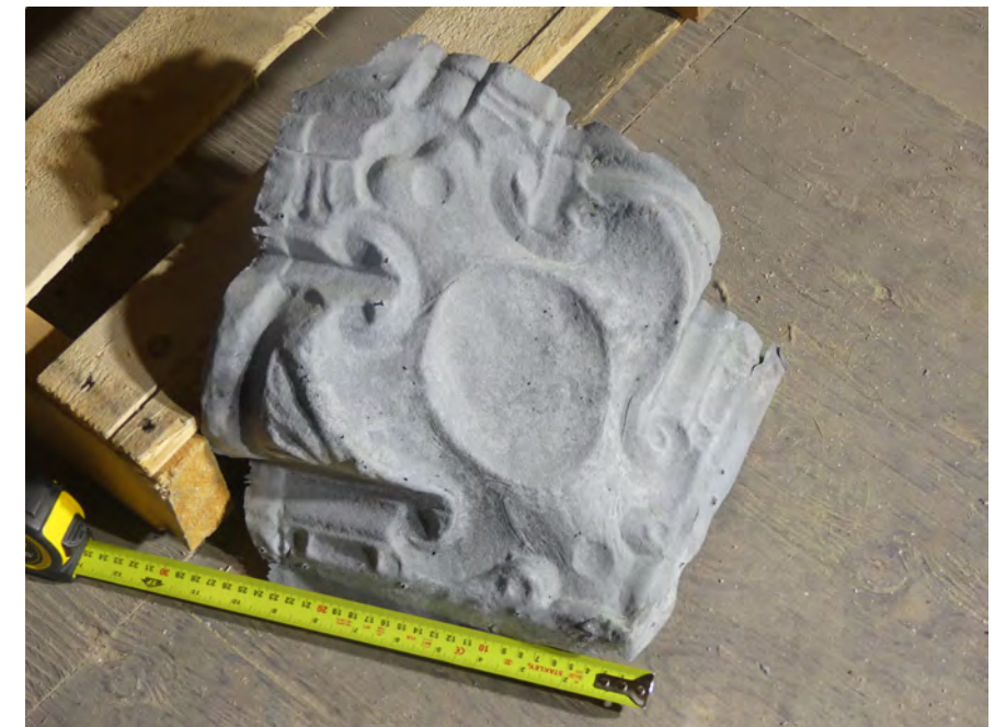
F. corner cornice piece: approx size 8" x 8" number required: 36 number available in usable condition: 8 replacement pieces required: 28
