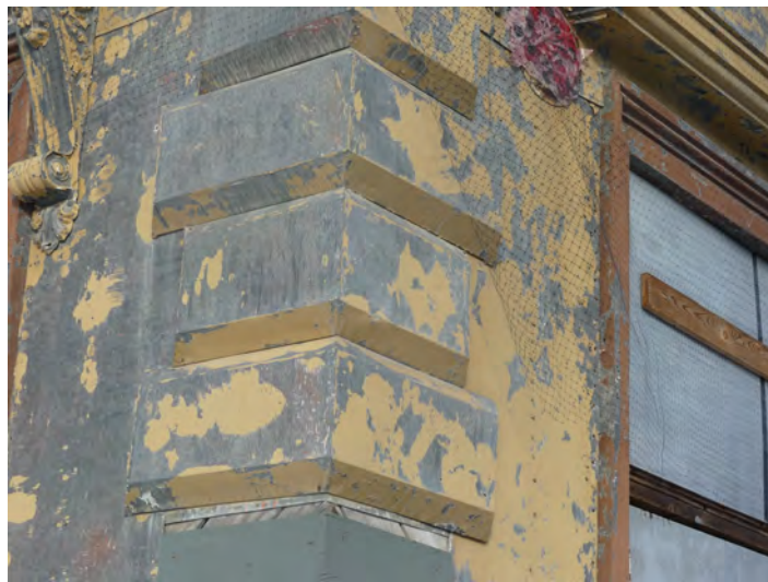
1. south east corner, quoins in typical alternating pattern. The outer corner is a folded joint, then with a mitred soldered joint top and bottom.
