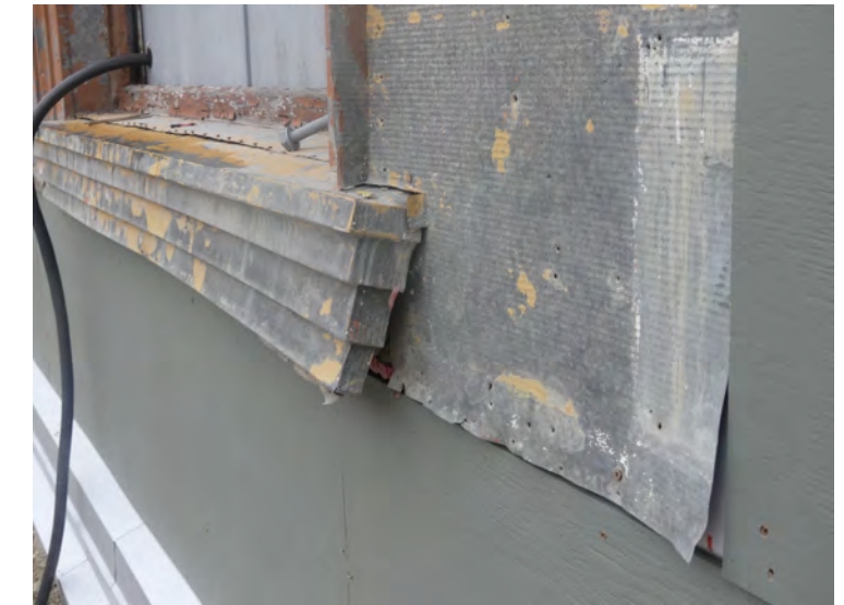
30. damaged sill, consider repair in situ. Typical metal siding panel, with rolled texture, replacement metal should retain this texture.
