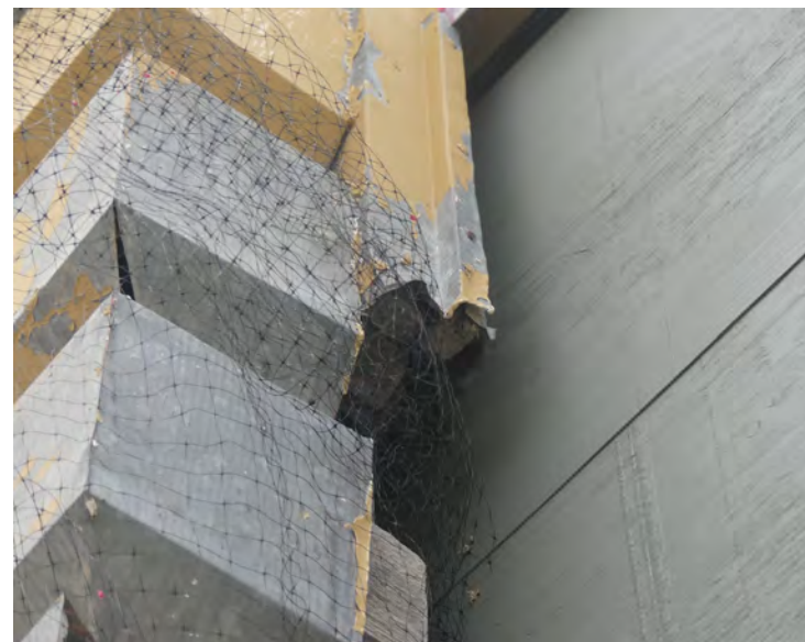
5. detail of area between existing metalwork and new stair. Detailing will be required for the connection. The open corner on the quoin, where the solder has broken, is typical in many areas
