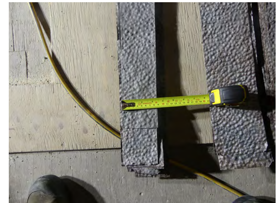
K: horizontal filler peice, between panels and cornice, variable widths and lengths to suit gaps. Virtually all pieces damaged, replace all replacement length required:
