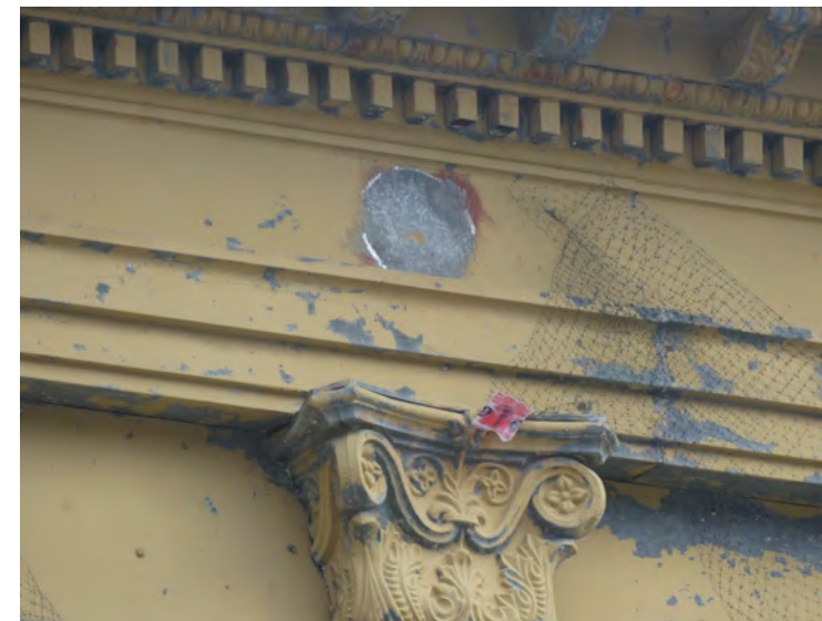
25. detail at location of missing medallion, 3 are missing on the north wall, 5 on the east wall
