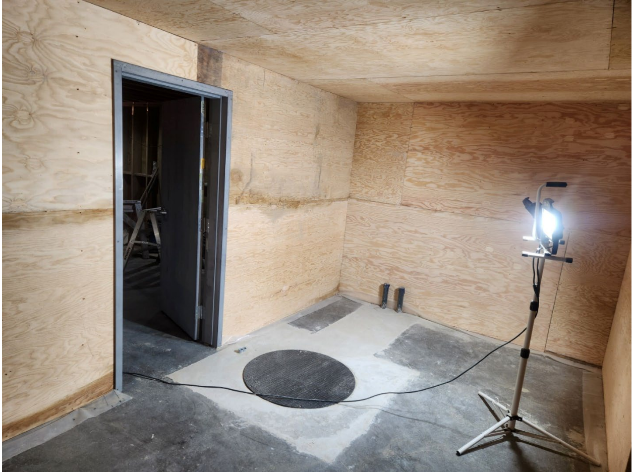
Figure 13: Sump pump room
