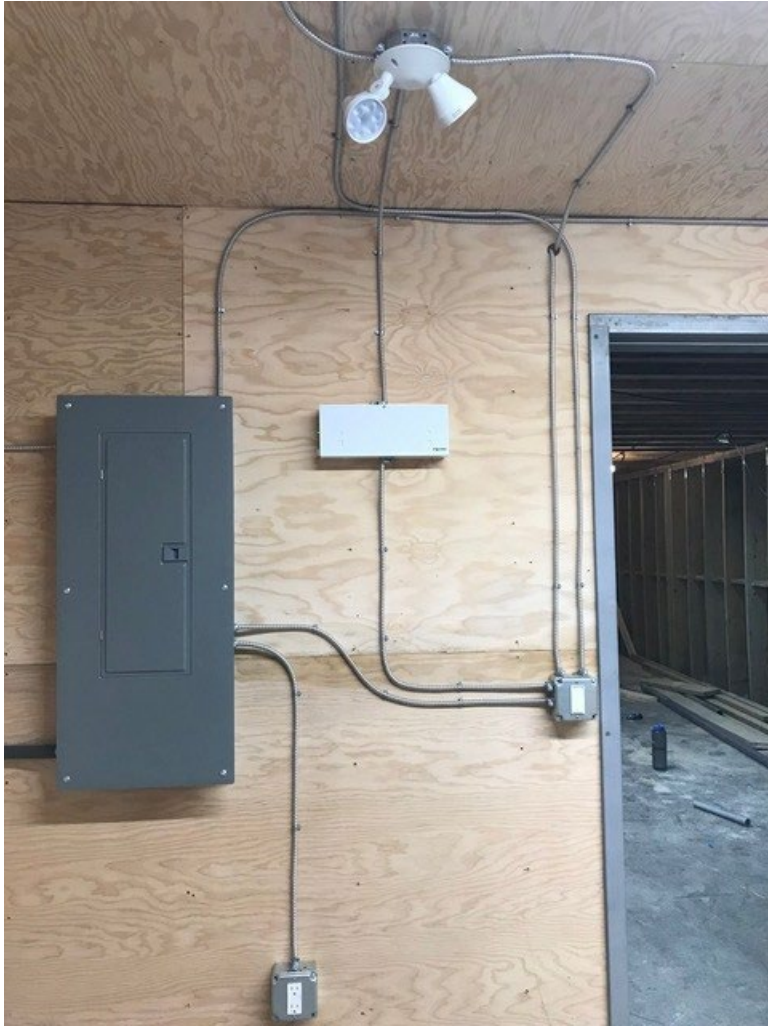
Figure 17: Electrical panel for lights, pumps, alarms
