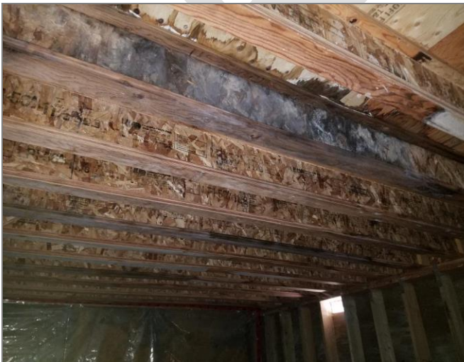
Figure 4.25 TJI showing deterioration at east elevation.
