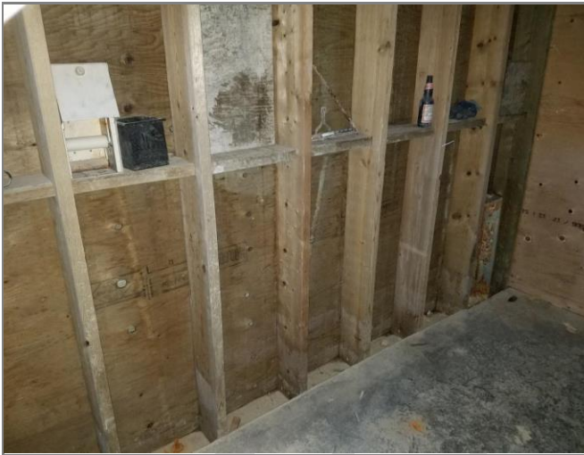
Figure 4.24 Basement framing (typ.) also showing water damage at sheathing north elevation
