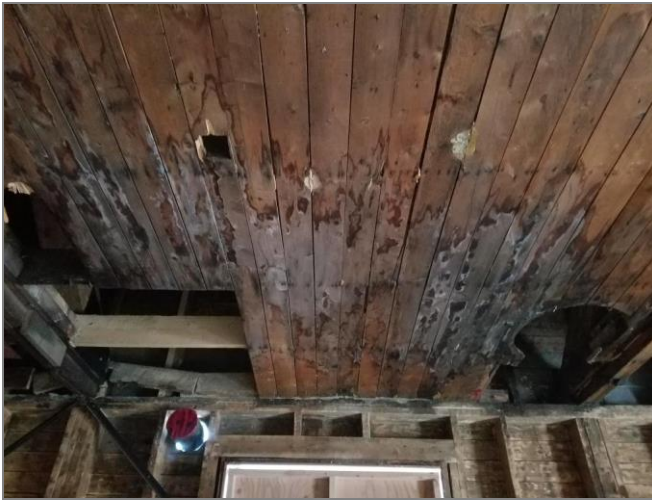
Figure 4.26 Second floor ceiling water damage/deterioration.
