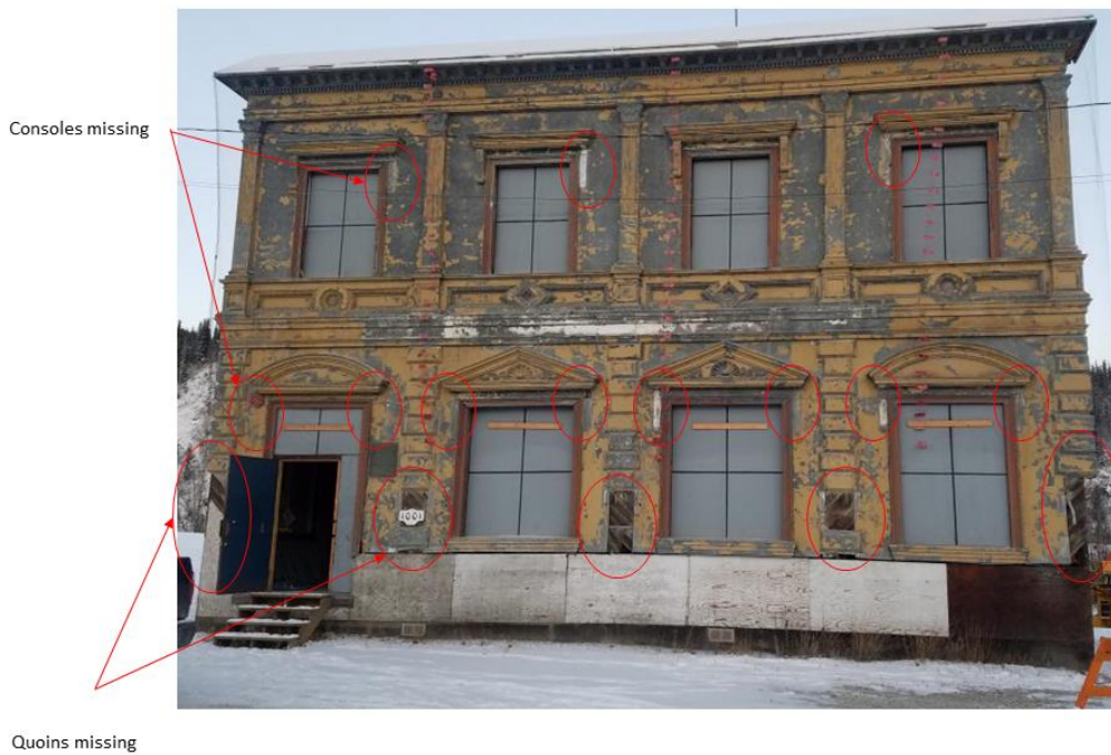
Figure 4.13 East elevation with damaged/missing cladding locations identified.
