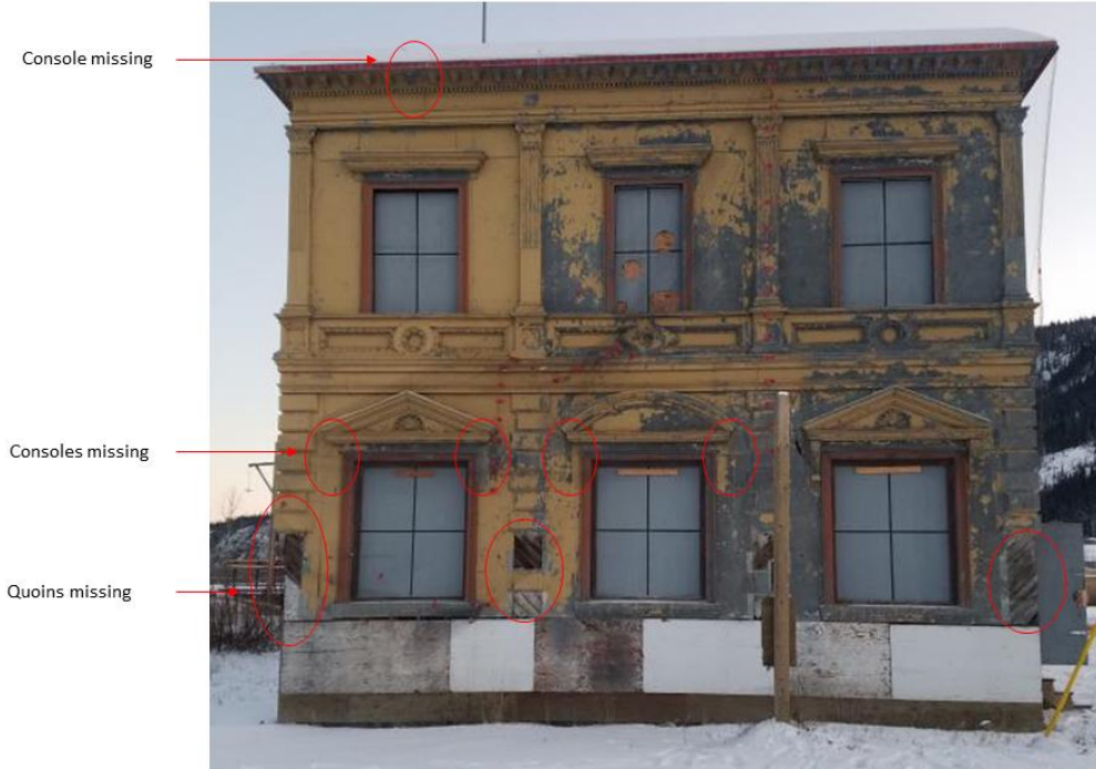
Figure 4.12 South elevation with damaged/missing cladding locations identified.
