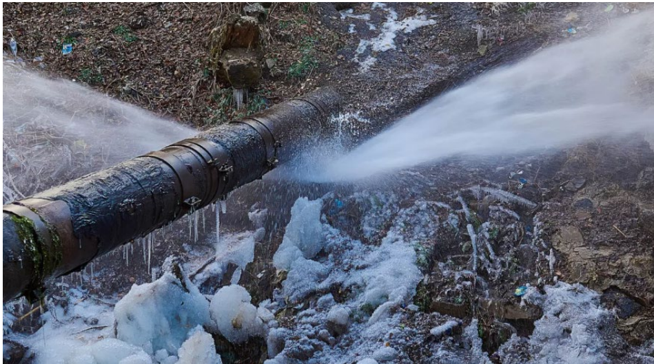
Watermain Break (Photo: City of Vaughan)
