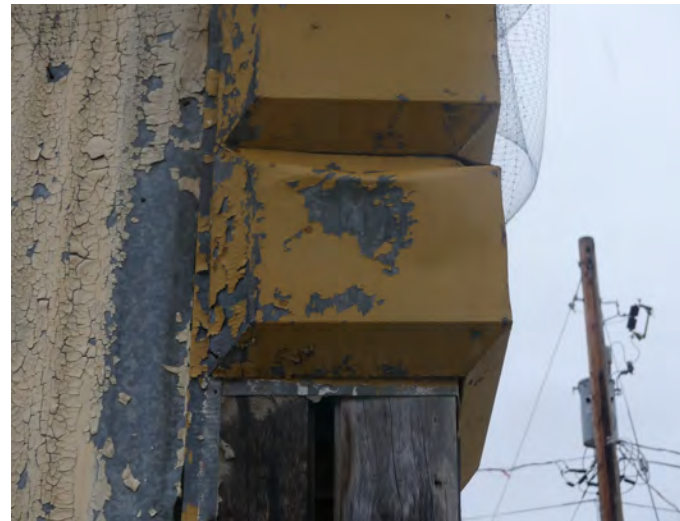
13. south west corner, some of the metalwork is damaged, repair would be feasible as this piece will be removed as a sample
