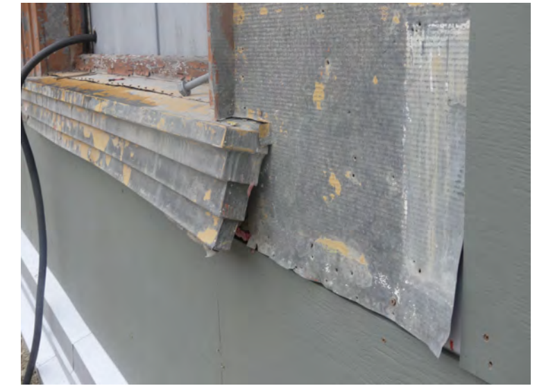
30. damaged sill, consider repair in situ, Typical metal siding panel, with rolled texture, replacement metal should retain this texture.
