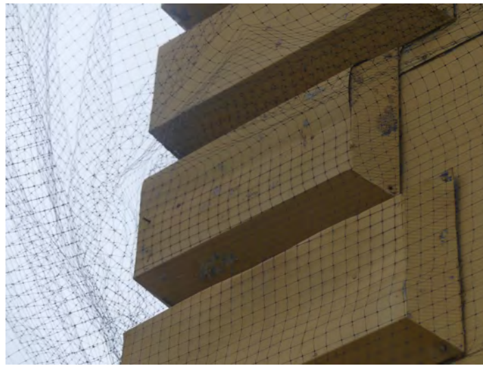
9. south west corner, typical metalwork, surface nailed to the metal substrate. Some damaged elements will need to be repaired or replaced
