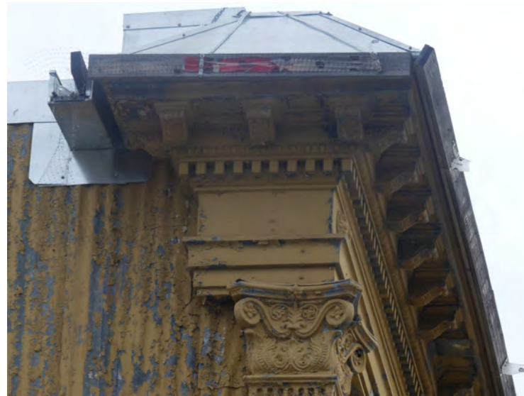
35. corner detail, note new scupper and temporary sloped parapet. Some joints have failed on the capital, and can be repaired in situ.
