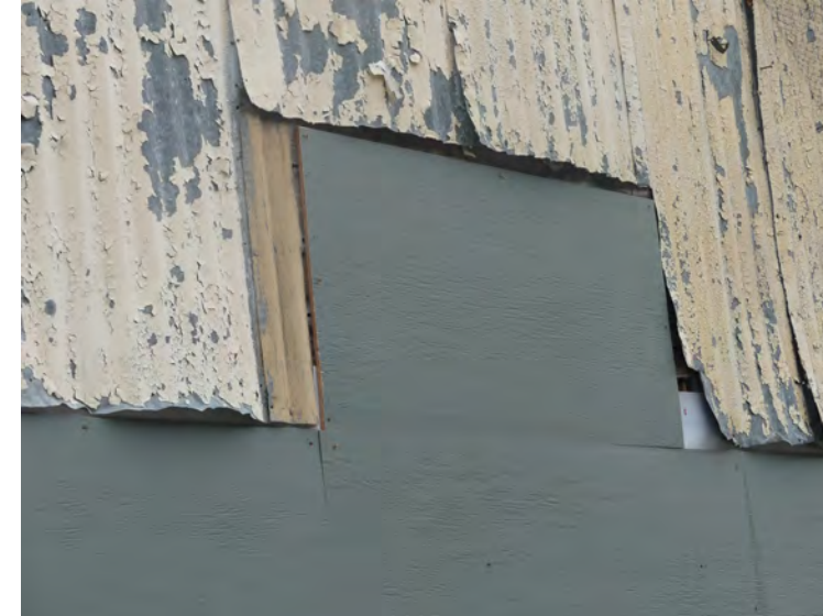
44. patch, archival photos show a door in this location which could be reinstated if desired. Typical siding will be scraped, refastened and repainted. The white finish is the suggested restoration color
