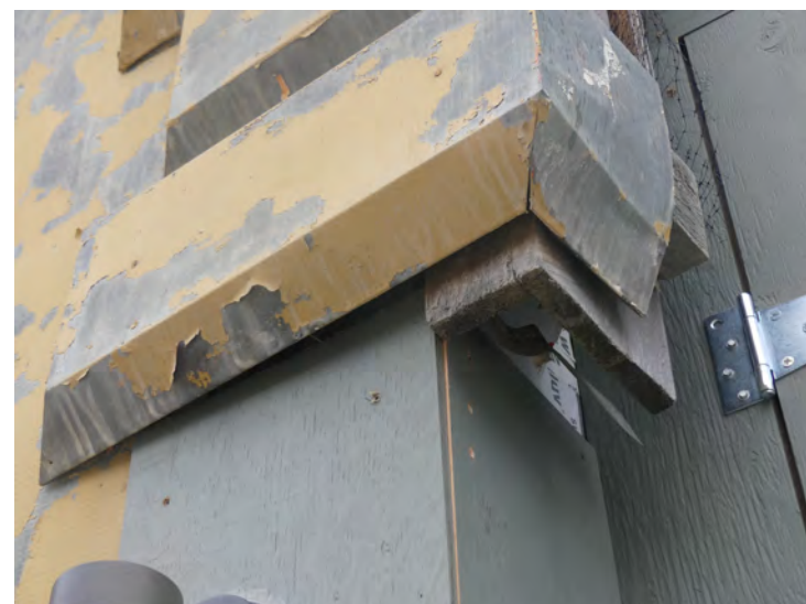
6. rough wood framing is installed under the metal for attachment and support
