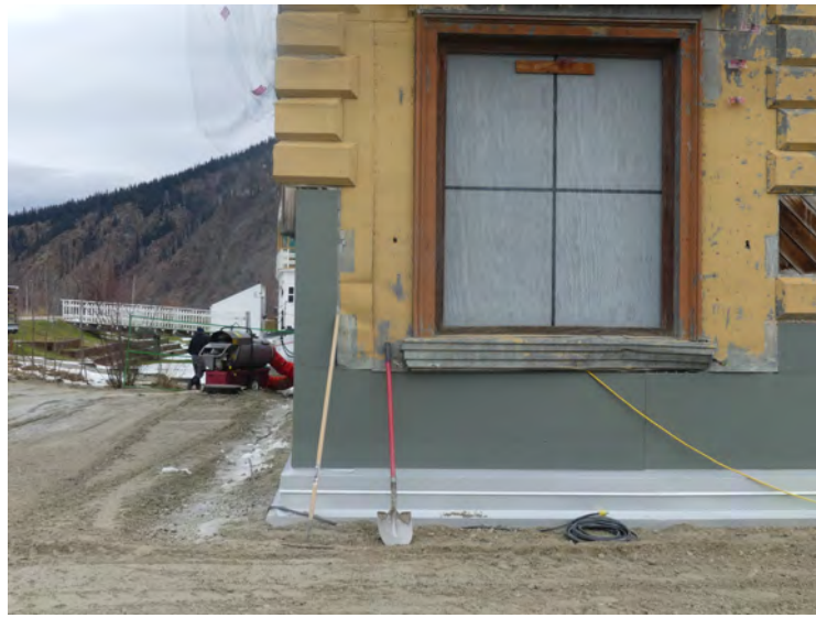
23. detail at corner, damaged sill and metal siding consisting of overlapping layers, nailed and with numerous penetrations
