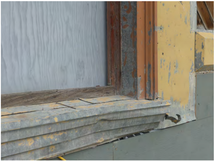
27. damaged sill, repair would likely require removal. Note the assembly with several pieces of overlapping metal. In some areas the sills fit around the siding, in others the siding runs beneath
