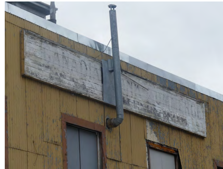
36. sign and stovepipe. The stovepipe should be retained as a historic element, the sign should be replicated and reinstalled, with the original stored as an artifact
