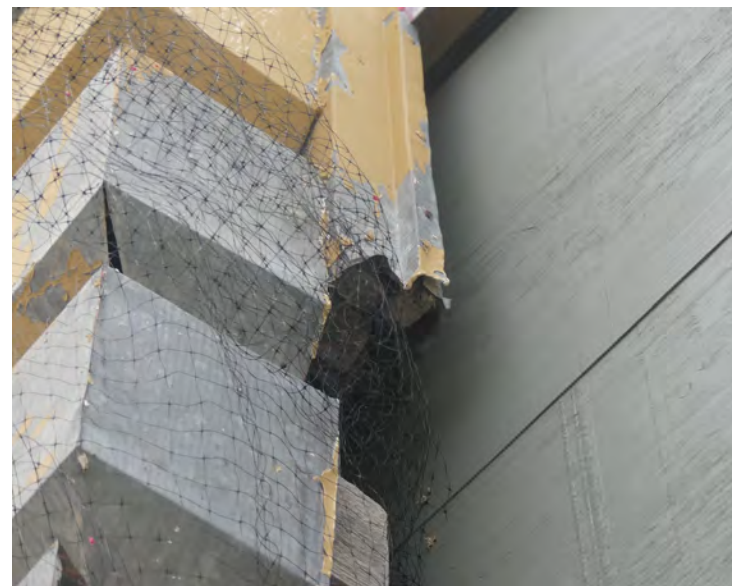
5. detail of area between existing metalwork and new stair. Detailing will be required for the connection. The open corner on the quoin, where the solder has broken, is typical in many areas
