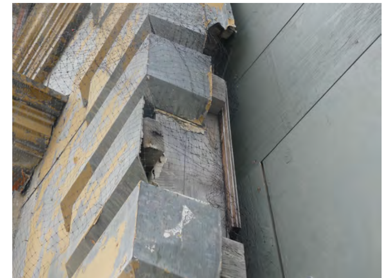
8. detail of damaged metalwork, to be made good. A sample of this corner detail should be removed and sent to be copied. Cladding details for the connection to the new construction will need to be developed
