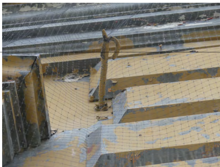
3. east wall, quins attached with galvanized roofing nails to the flat galvanized metal substrate. They are installed without flanges, although some areas show a metal plate between. The hook is for an early wiring attachment to the building, and could be retained
