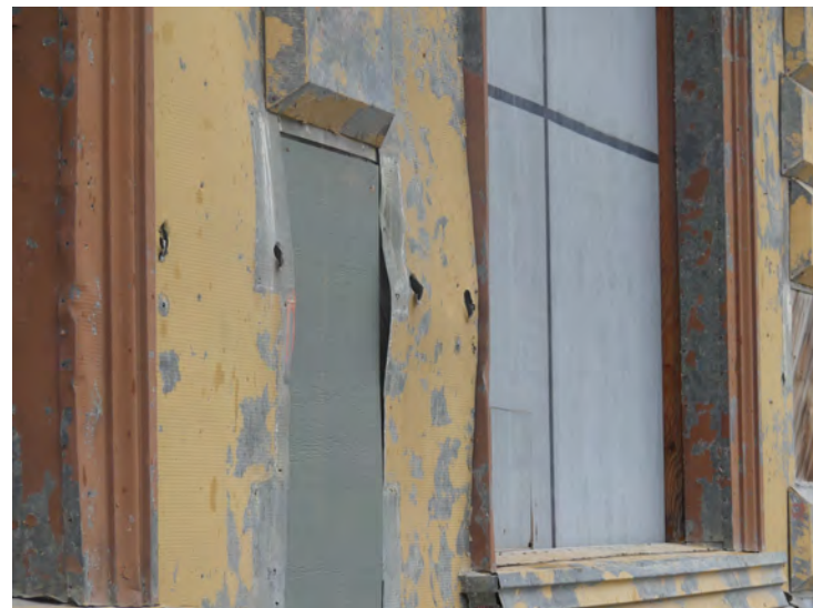
20. area adjacent to entry door, damaged metal molding for door frame, holes in metal siding, damaged sill. This also shows the metal filler strip between each quoin
