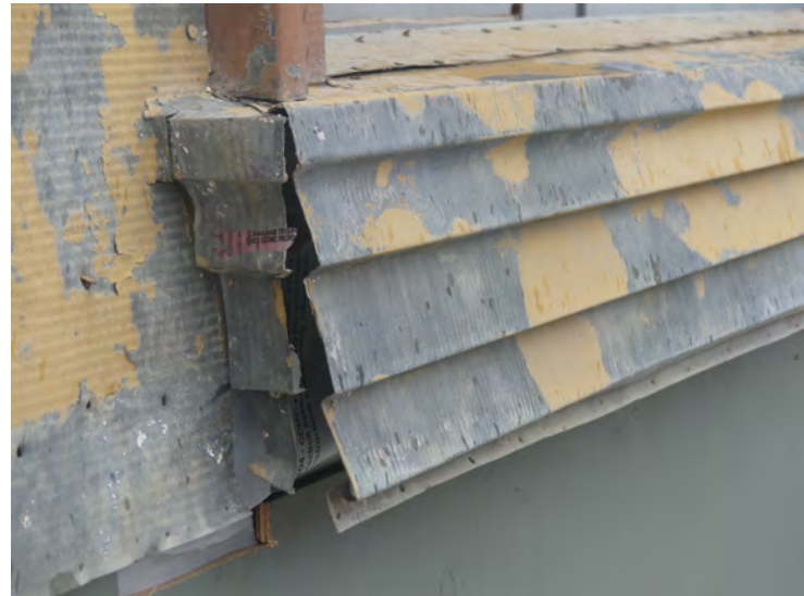
21. the lower windows sills are generally damaged from when the building was raised. Repair or replacement of the sills will require careful disassembly of the adjacent metal siding. Some sills may be repairable in place and resoldered.
