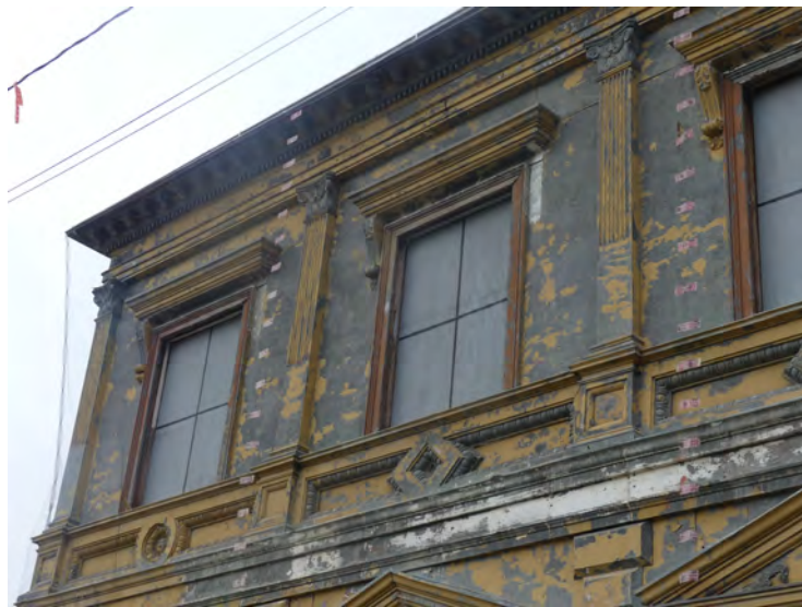
15. upper wall, generally intact, some quoins missing, The original paint color shows where the sign was located
