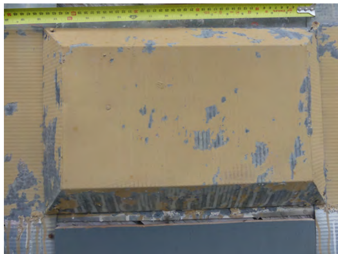
11. the quoin below has been removed, the horizontal transition strips and the condition of typical siding show clearly. Renailing and filling of mail holes and other penetrations will be required
