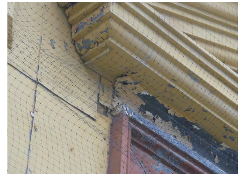
26. detail at window head, metal siding panels to be reattached and repainted
