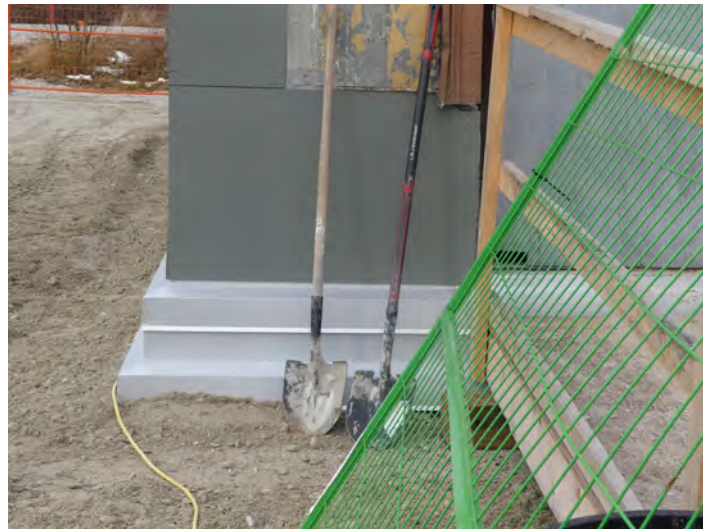
19. east wall, strip view showing new step flashing and extent of quoin replacement, final grade to be confirmed
