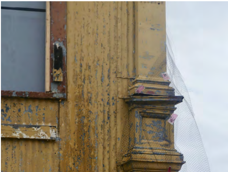
39. south west corner, detail of siding and metal capital. The siding on this elevation consists of several smaller panels, retaining these would be part of the restoration process
