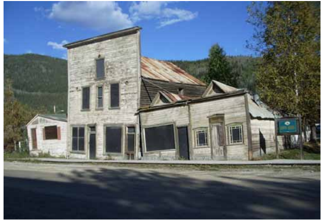
The Third Avenue complex, owned by Parks Canada, contributes to the sense of decay that characterizes much of Dawson. (Photo: H. Kalman)
