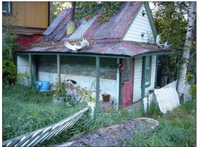
This small cottage and its fence have become derelict and the garden is overgrown. They provide an effective photo opportunity and contribute to Dawson's texture, but will collapse if left unmaintained. They should be stabilized and preserved, following the Standards and Guidelines for the Conservation of Historic Places in Canada. (Photo: John Stewart)
